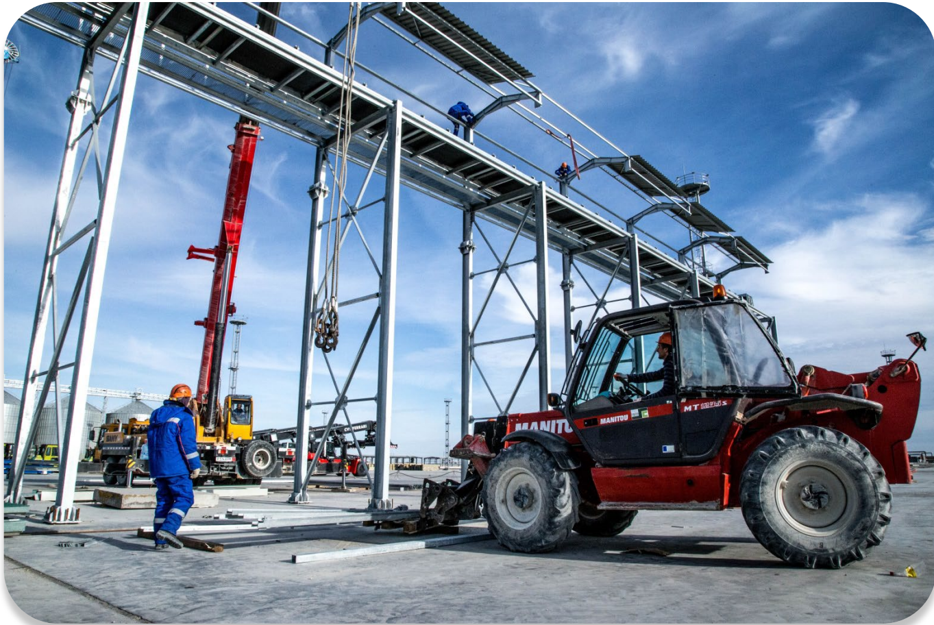
Support structure for 500 t/h belt conveyor with mobile tripper
