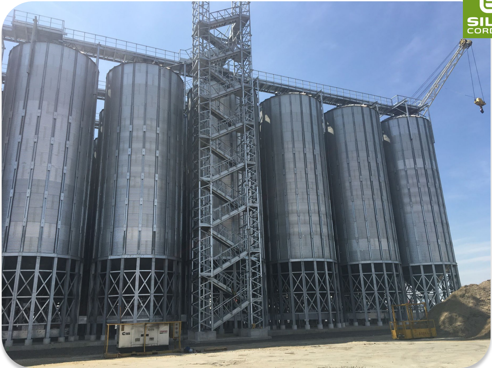
2018 GRAIN TERMINAL ANTWERP – BELGIUM : 37 Hopper silos mod. 7,64/16 45° – Total capacity: 20,000 T
