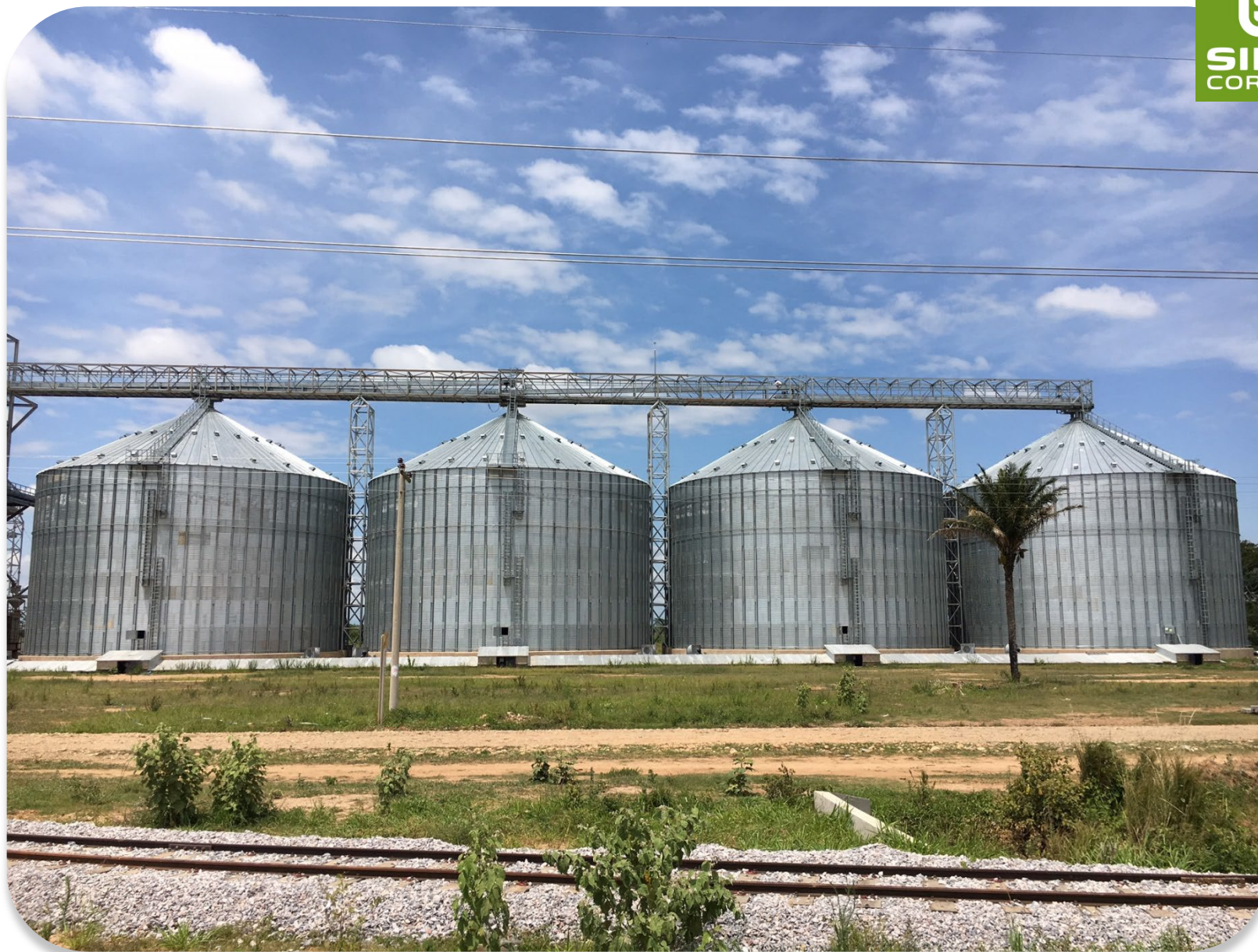
2016 OMEGA - BOLIVIA: 4 silos mod. 27,50/20 – 4 silos mod. 7,64/13 - Total capacity: 36.000 T
